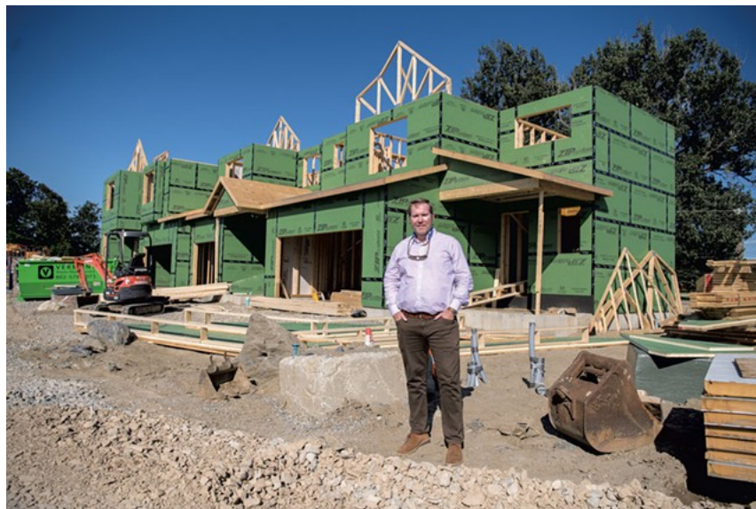
Above: O'Brien Brothers CEO Evan Langfeldt at the construction site of Hillside East in South Burlington
